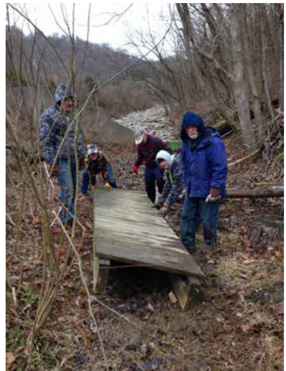
Volunteers putting the Eagle Scout Bridge back into place on Bender Mountain after a winter storm.
